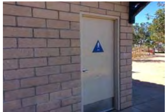
Photo #12: Hollow metal exterior door
