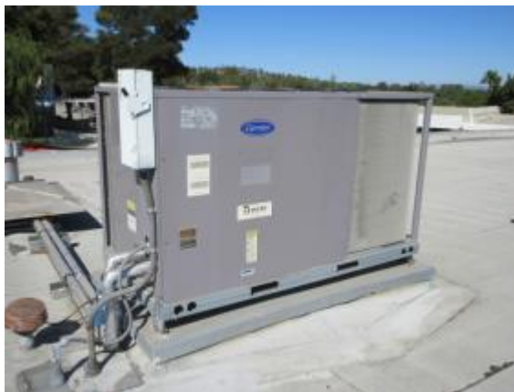
Photo #29: MPR condensing unit
