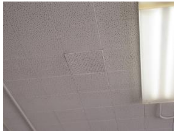
Photo #40: Loose ceiling tiles
