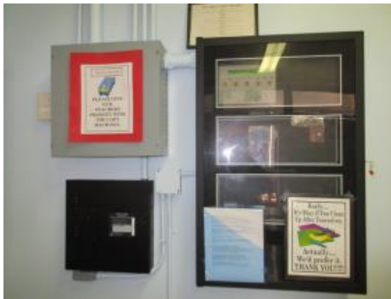
Photo #27: Fire alarm
