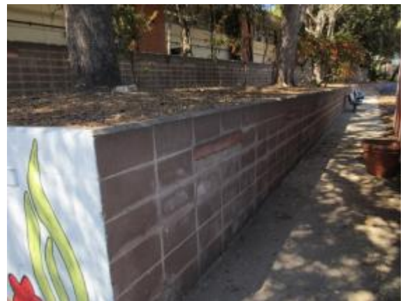
Photo #42: Efflorescence at retaining wall
