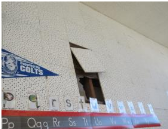
Photo #39: Missing wall (clerestory) tiles
