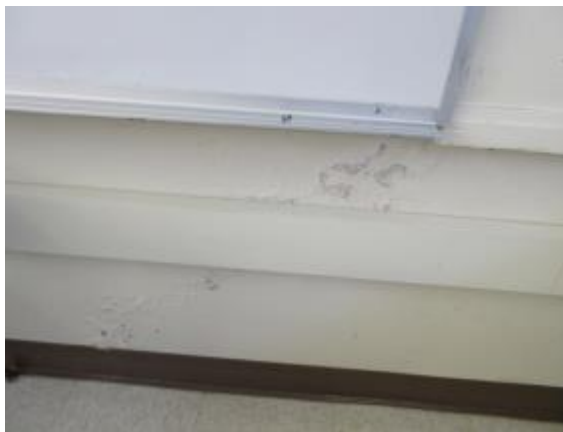
Photo #41: Water damage at Classroom 21
