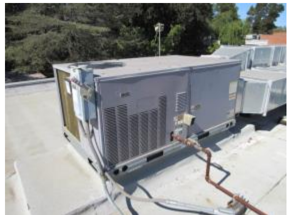
Photo #30: Rooftop package unit
