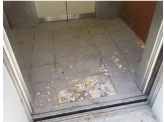
Photo #38: Damaged floor tiles at elevator cab
