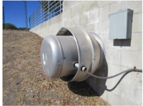
Photo #26: Elevator equipment room exhaust fan
