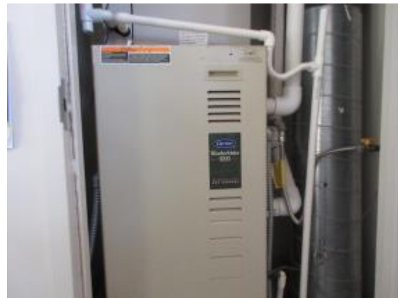
Photo #28: Gas furnace
