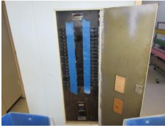
Photo #37: Abandoned in place electrical panel
