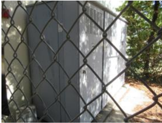
Photo #25: Main switchgear
