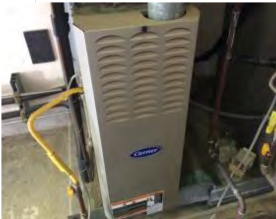
Photo #27: Gas furnace
