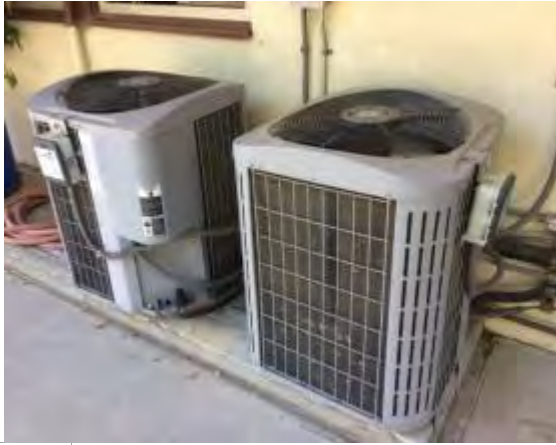
Photo #25: Condensing units
