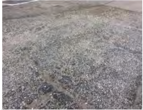
Photo #8: Parking lot with damaged asphalt
