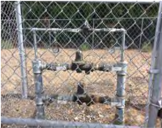
Photo #33: Backflow preventer
