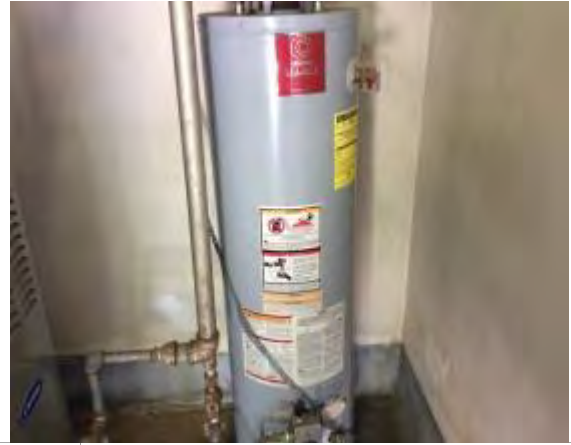
Photo #26: Water heater
