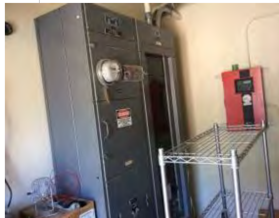
Photo #30: Main switchboard
