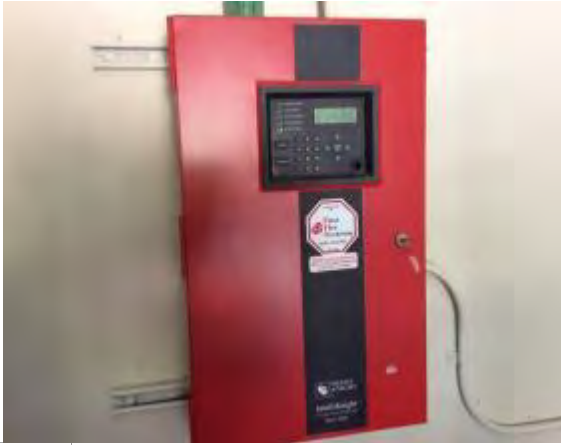
Photo #31: Fire alarm control panel
